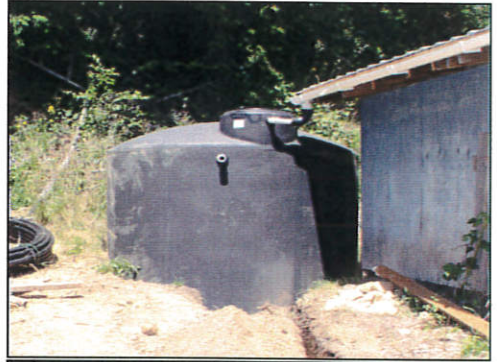
Roof rainwater collection (via roof gutters connected to 3,000 gallon collection tank and gravity fed pipeline to stock waterers) provides alternative off-stream water source for livestock
