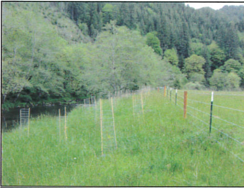
Exclusion fencing installed and riparian areas planted along pasture (Lower Big Elk) for future shade and woody debris inputs to the aquatic system
