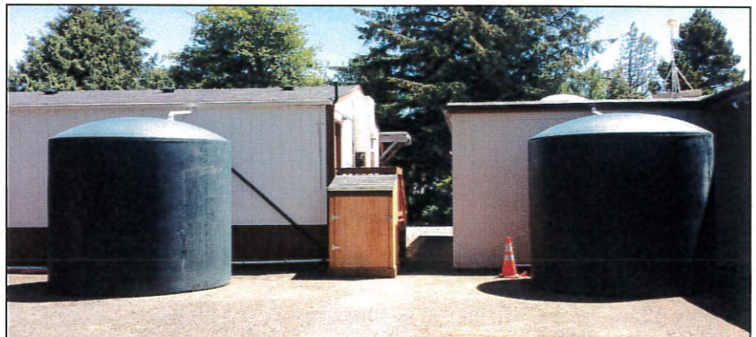
Two 5,000 gallon rainwater collection cisterns and a pump house collect rain water from the Pantry and church roof and delivers it to the garden.
