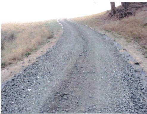
Resurfaced forest access road reduces sediment to local streams in Big Elk Creek
