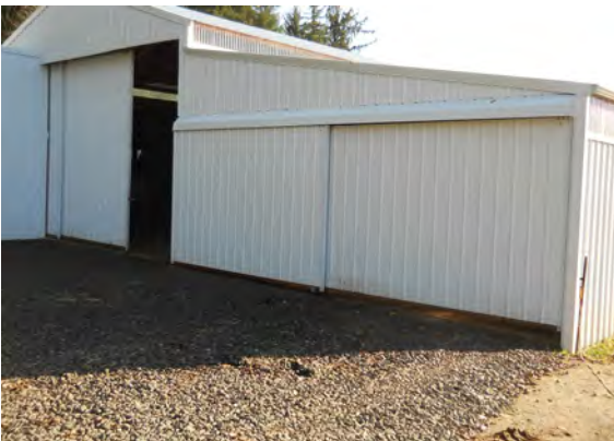
Best management project featuring gutters for stormwater management and gravel for mud control, BMPs like these prevent unnatural levels of sediment and possibly bacteria from entering public waters
