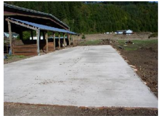
Concrete slab in an area of heavy use to prevent accumulation of mud.
